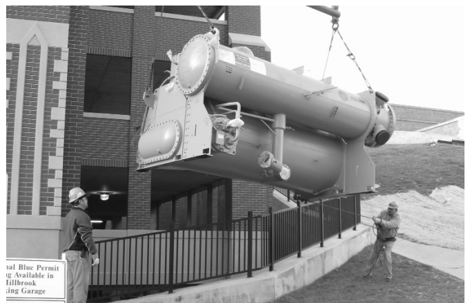
▲ Haberberger lowers the 700-ton chiller's main section into the sub-grade garage at Washington University Village East.
