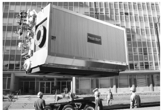
▲ Haberberger's crew hoists Boiler #6 over the Scott Avenue Pedestrian Bridge at the Washington University School of Medicine. Pictured: Terry Gibson, Tim Gallagher, Ed Quinn, Chad Huff, Dan Daniels and Andy Finklang. Not pictured: Frank Herrell.
