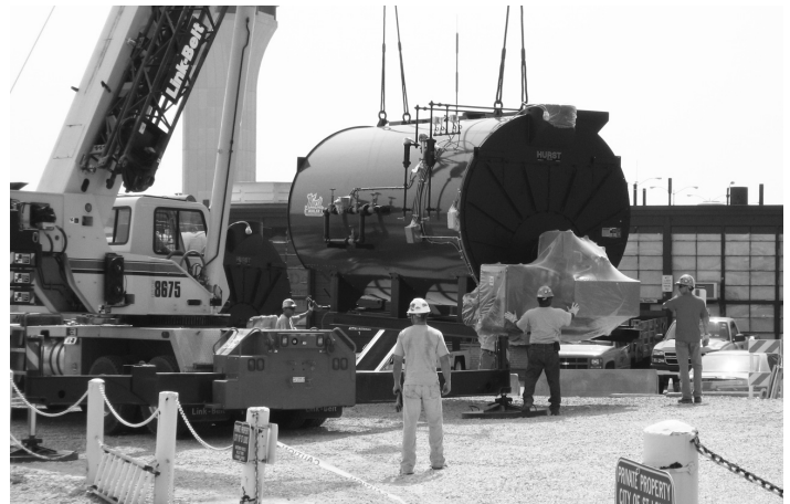
▲ Haberberger workers (from left to right) Charlie Bott, John Boyd and Dave Walther hoist a 750 HP boiler onto a truck as a Taylor Excavating employee (foreground) looks on. The boiler was then transported to the Airport West Plant for installation.
