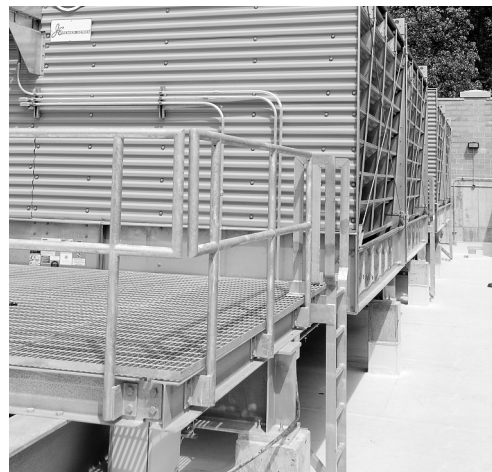
◀ The four 550-ton cooling towers, which were installed by Haberberger's crew, are pictured.
