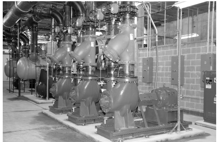
▲ Three condenser water pumps (foreground) and two chillers (background) are pictured above.
