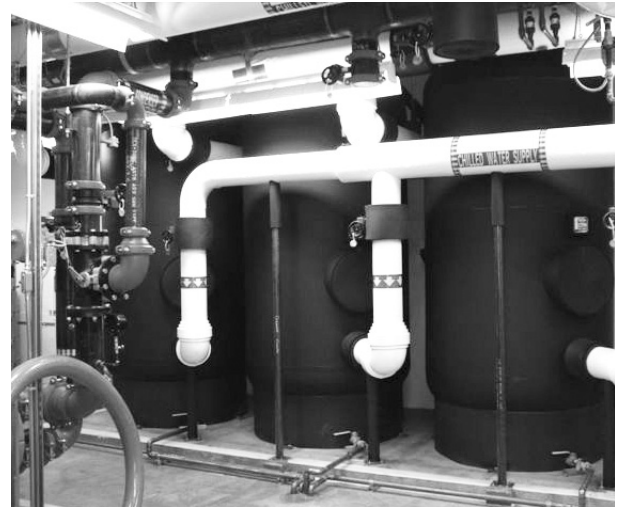
▲ The three chilled water storage tanks at the Washington University Genome Data Center are pictured above.
