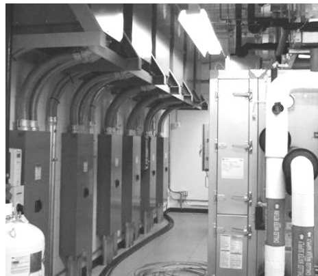
▲ One of the four main Air Handling Units is pictured above at the Washington University Genome Data Center.
