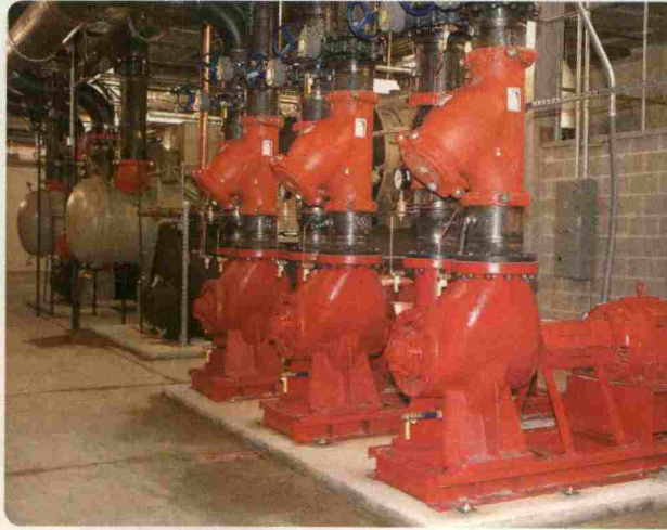
Condenser water pumps installed by Haberberger at Washington University. Photos courtesy Haberberger
